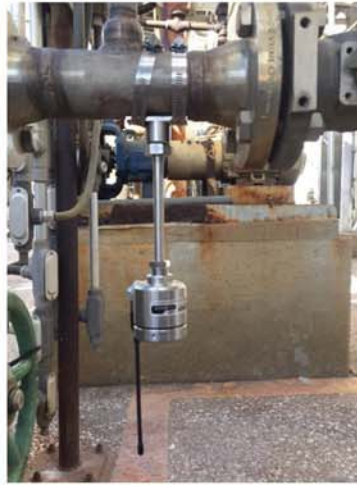
High-temp dual-element unit installed using pipe bands.
