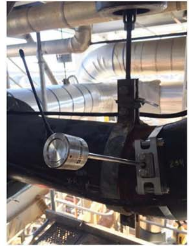
Ultra-high-temp unit installed using pipe clamp.
